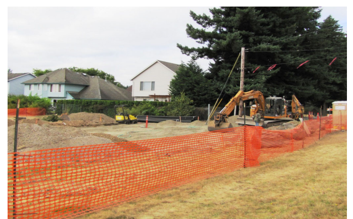
Construction of two parking lots at Sunrise Park will be completed by the end of September.
